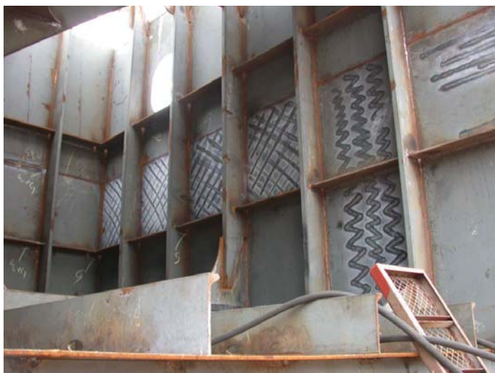
Photograph 12-7. Shop primed block showing corrosion of edges and welds and zinc corrosion products at sites of burn through and fairing processes.
