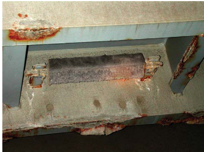
Photograph 6-5. Poorly sited anode, the anode is enclosed and can only protect a small area.
