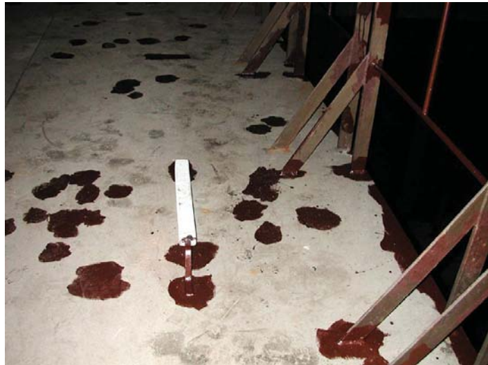
Photograph 5-1. Brush applied touch up paint on a forepeak stringer.
