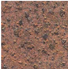
Rust Grade D
