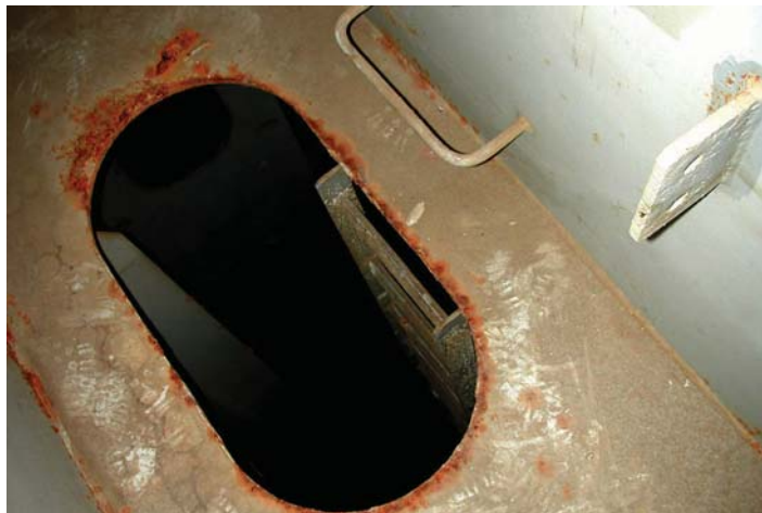
Photograph 12-15. Coating breakdown around cut out.
