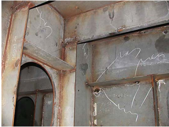
Photograph 12-8. Corrosion at all the welds and edges of a shop primed block. Note also the presence of welding fume, chalk marks and oil contamination.
