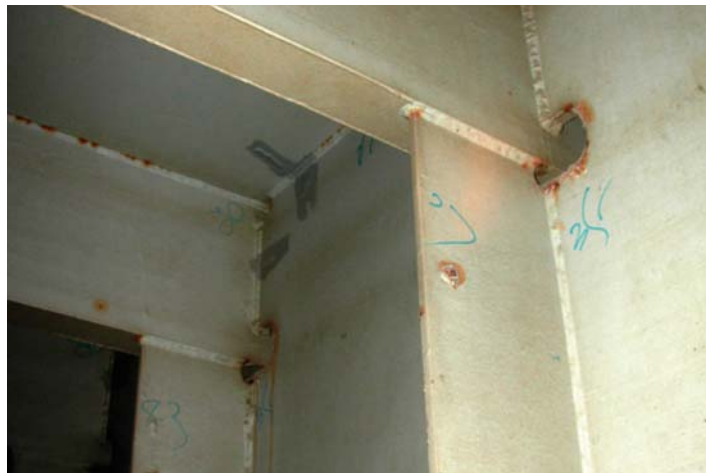
Photograph 12-26. Stress corrosion at cut outs.
