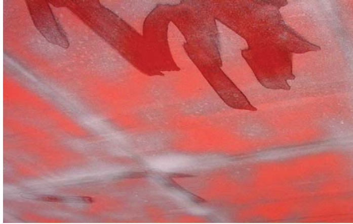
Photograph 4-3. Poor removal of oil contamination using solvent and a brush. The dark area at the top of the photograph shows the extent of oil contamination after cleaning.
