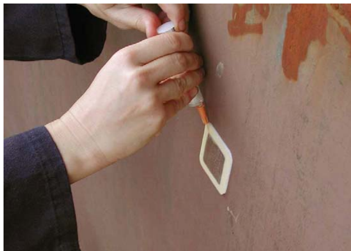
Photograph 4-5. Salt contamination testing.
