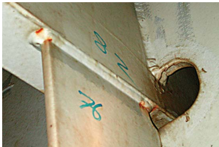
Photograph 12-27. Stress induced corrosion at toes of welds.
