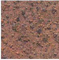
Rust Grade D
