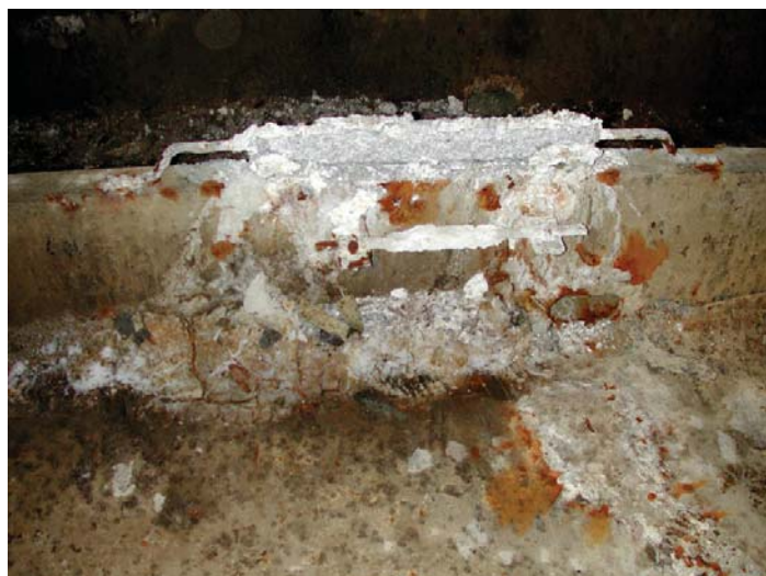
Photograph 6-2. Overworked zinc anode.
