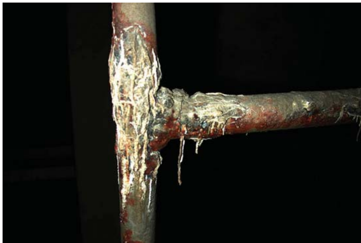
Photograph 12-19. Voluminous calcareous deposits.
