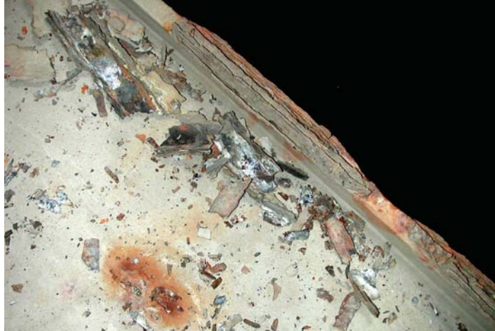
Photograph 12-14. Coating breakdown on stiffener edge.
