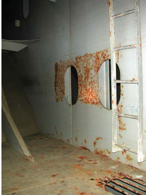
Photograph 12-20. Example of poor surface preparation prior to coating.
