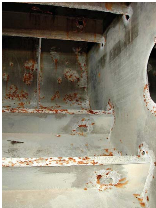
Photograph 6-4. Heavy calcareous deposits.
