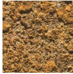
Rust Grade D
