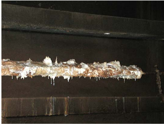
Photograph 6-3. Overworked aluminum anode.
