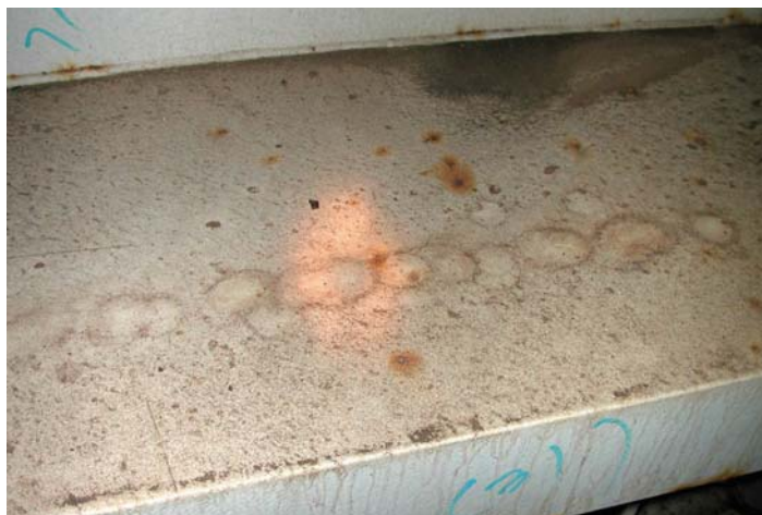
Photograph 12-10. Corrosion spots on longitudinal stiffener.
