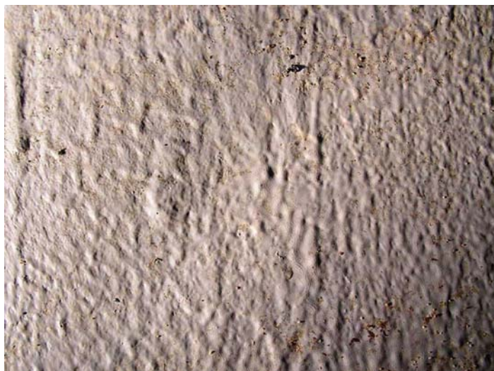
Photograph 12-1. Poor coating application control.
