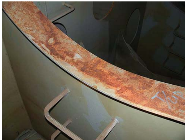
Photograph 12-4. Where the coating is too thin, early failure occurs in service.
