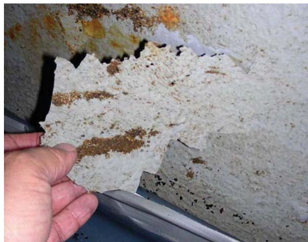
Photograph 12-3. Over thick coating detaches easily. Poor preparation between coats of paints causes early failure.
