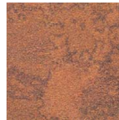
C HB 2 H Heavy Flash Rusting
