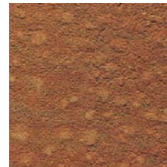
D HB 2 H Heavy Flash Rusting
