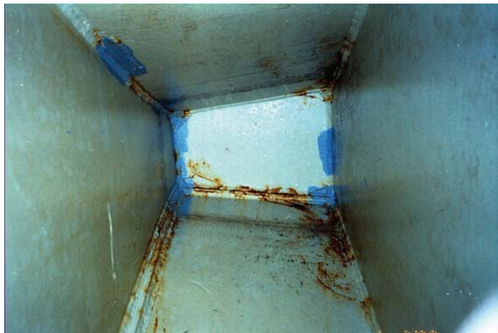
Photograph 12-17. Corrosion at welds.
