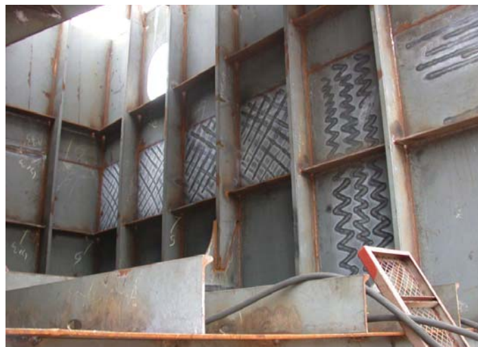
Photograph 8-3. Shop primed block showing corrosion of edges and welds and zinc corrosion products at sites of burn through and fairing processes.
