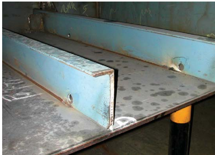
Photograph 4-2. Oil and grease stain stains during block assembly show as dark stains on the shop primer.
