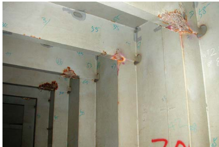
Photograph 12-25. Stress-induced coating failure.
