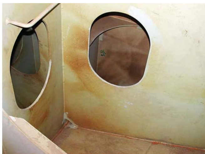
Photograph 12-5. Trapped grit at the welds and in the coating has caused rust staining. Grit that penetrates through the coating will allow corrosion of the substrate to initiate.
