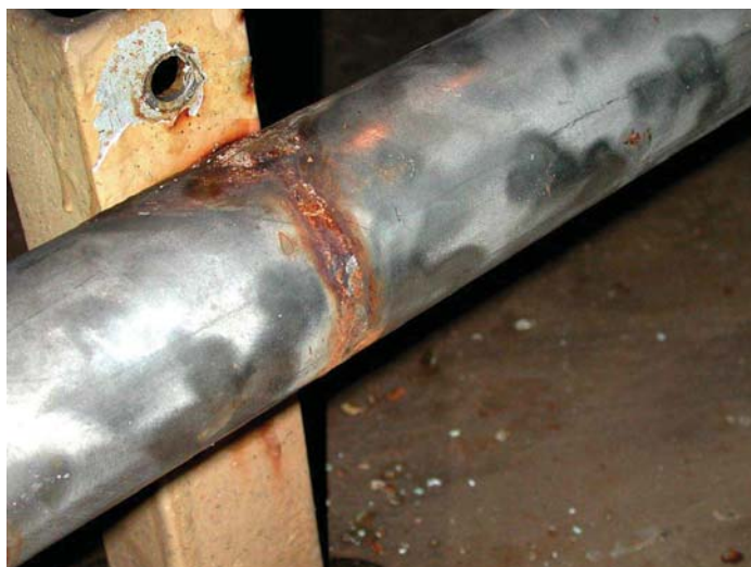
Photograph 1-2. Pits forming as a result of crevice corrosion between the U bolt support and the pipe.
