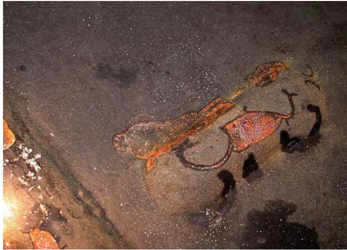
Photograph 1-4. Structures in way of tank washing systems can lose their coating and pitting corrosion can occur.
