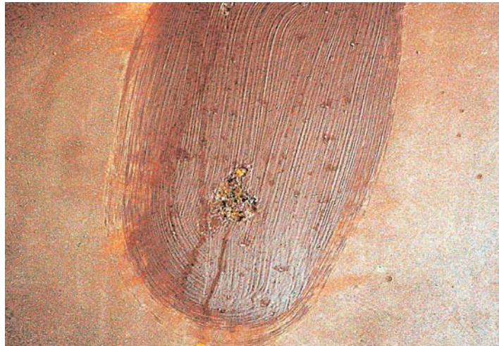
Photograph 3-1. Localized repair in this coating has failed again at the same site.
