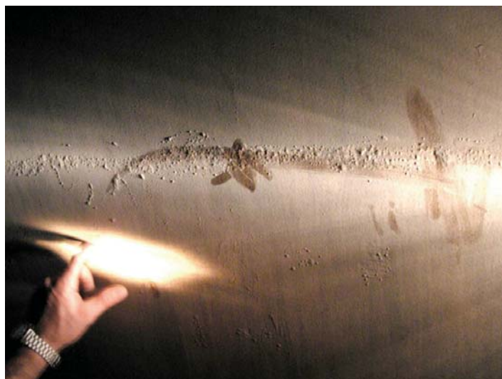
Photograph 4-10. Blistering where a stiffener was welded on the other side of the plate.
