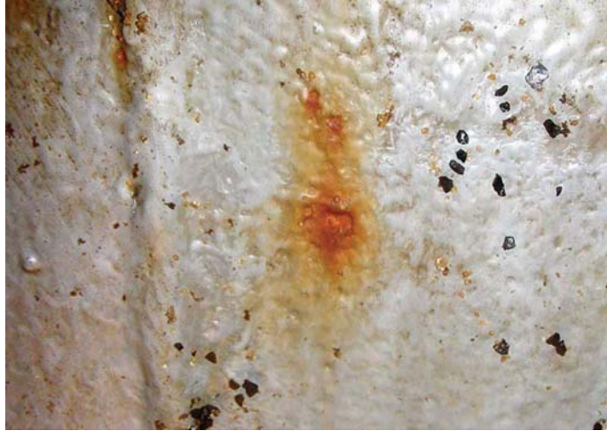
Photograph 12-2. Small holes or holidays in the coating allow rapid corrosion to initiate in service.
