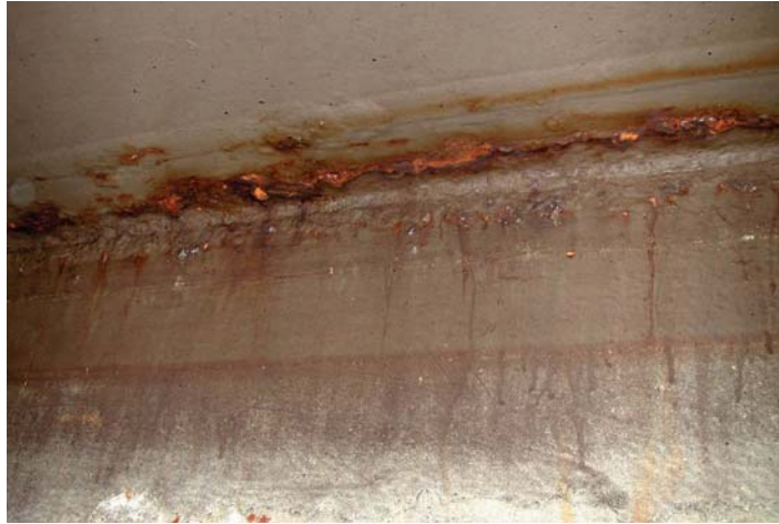
Photograph 12-16. Corrosion around weld.
