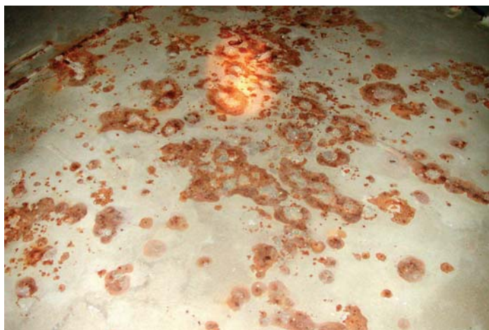
Photograph 12-11. Corrosion spots on stringer deck.
