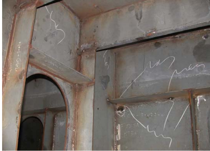
Photograph 8-4. Block stage with shop primer, prior to secondary surface preparation. Note the corrosion at all the welds and edges and the presence of welding fume, chalk marks and oil contamination.
