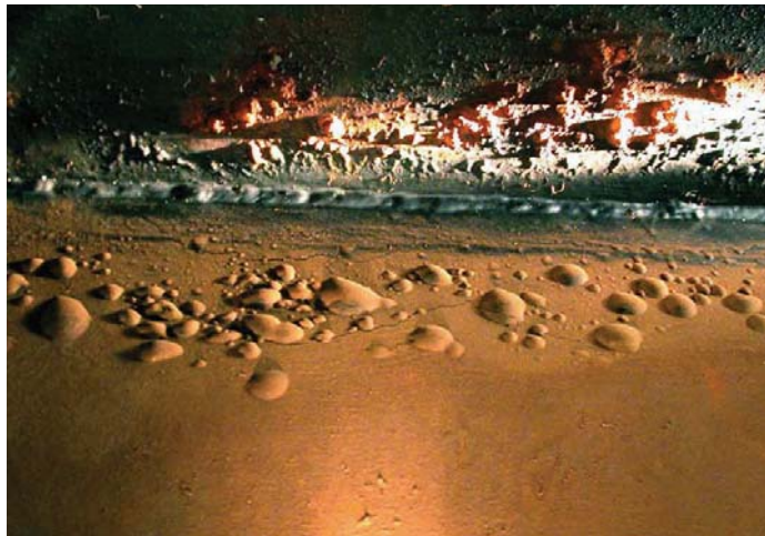
Photograph 1-1. Cathodic blisters surrounding an active anodic site.
