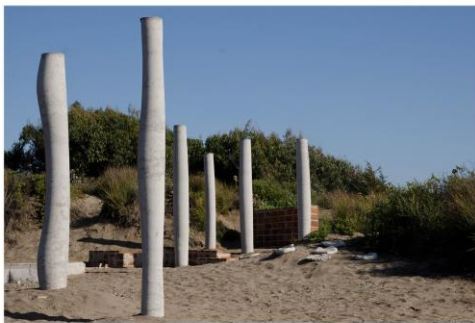
Columns are a basic architectural element: with flexible formwork it is possible to achieve new forms for them.
